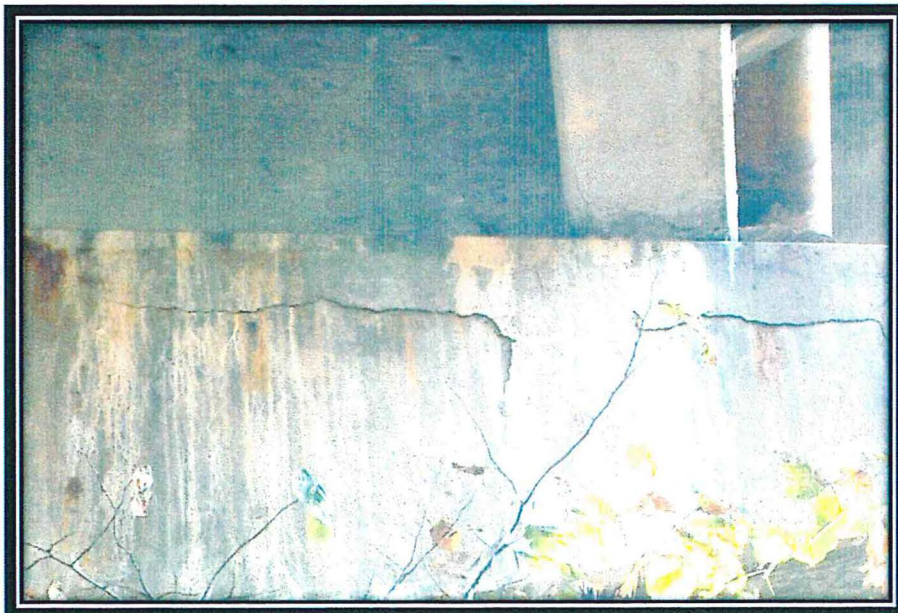
Cracks on West Pier Cap
