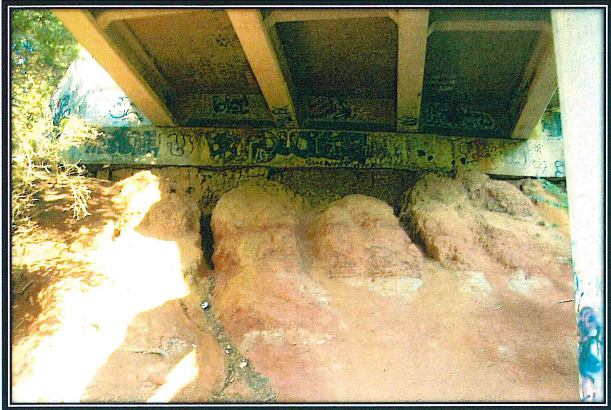
Erosion at East Abutment, West is similar
