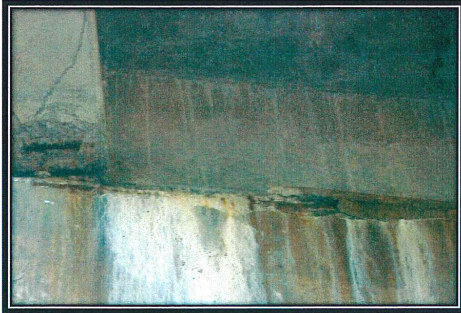
Spalling and Staining on Pier Cap
