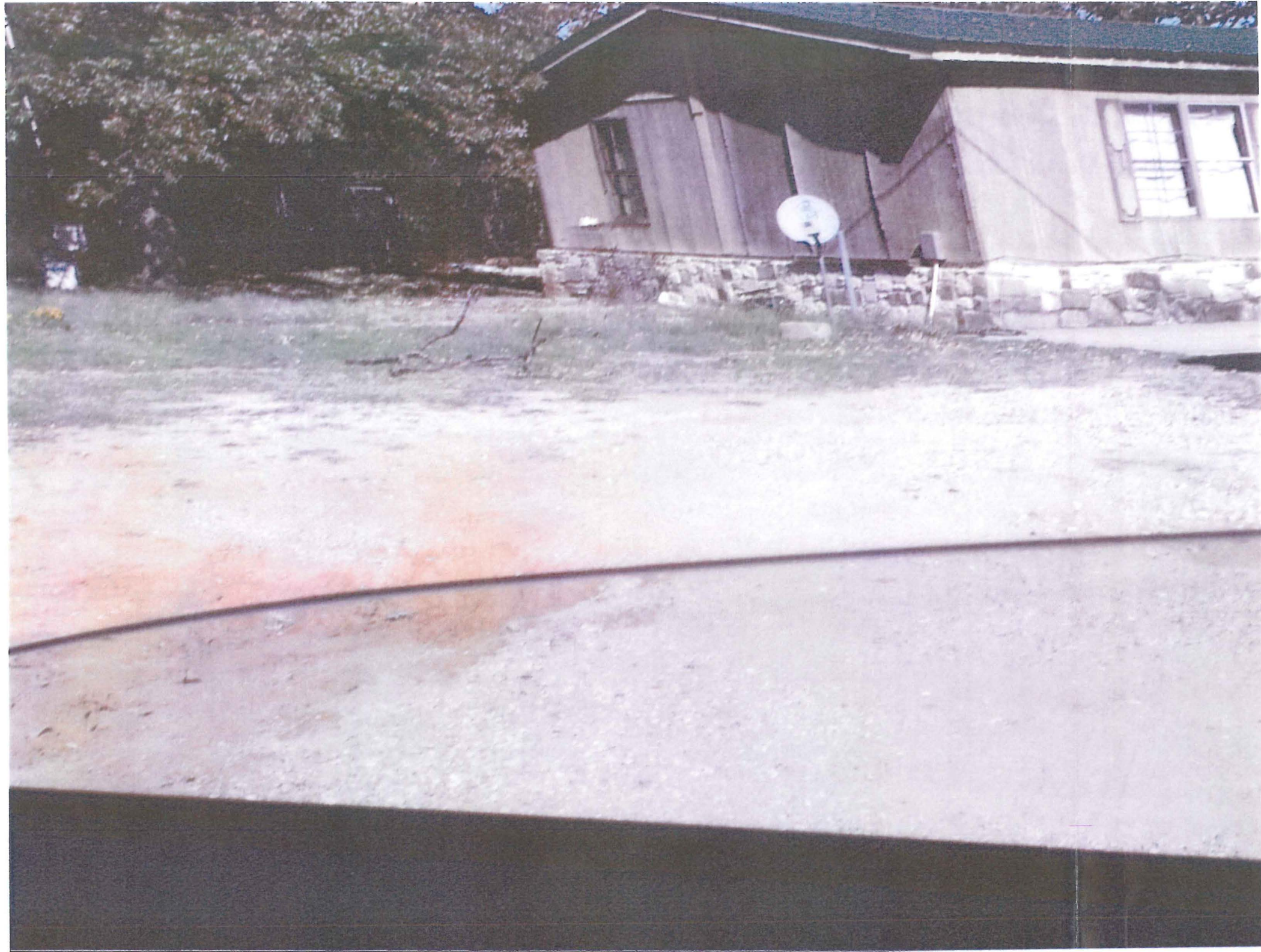
Falling apart Permanent structure
