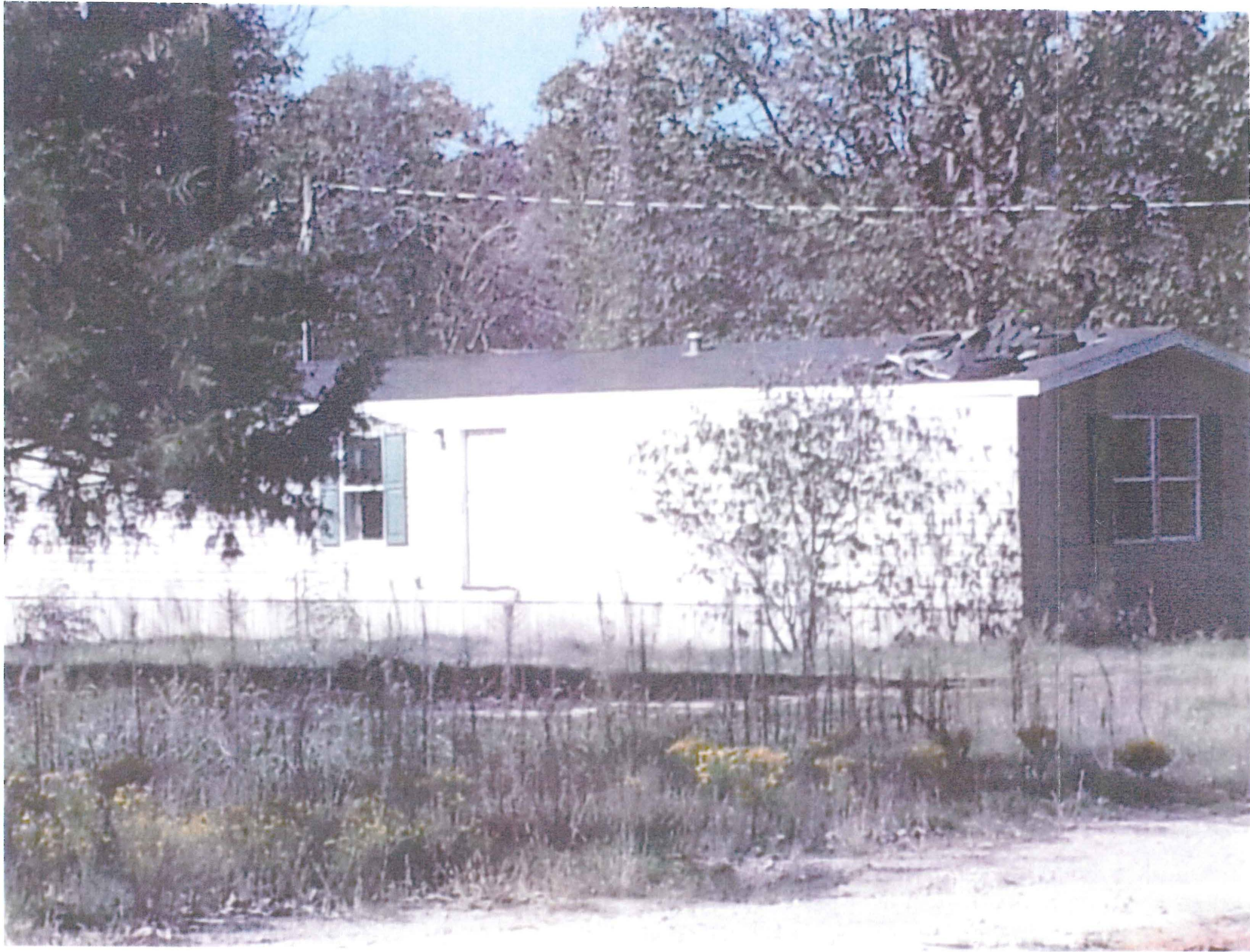
Not moved Tires holding down tarp on roof
