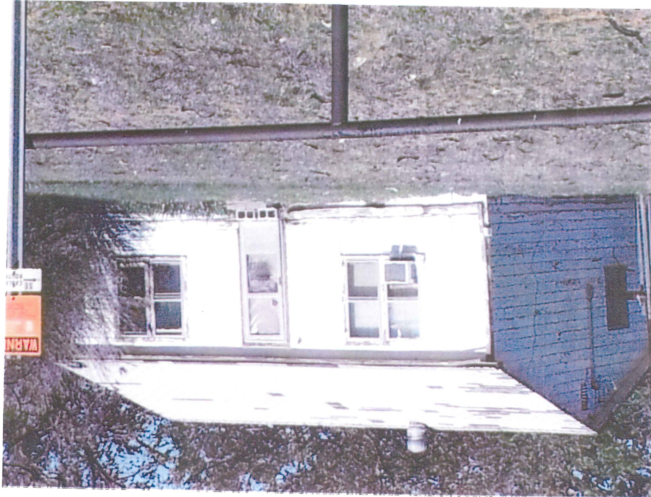
Permanent structure falling apart
