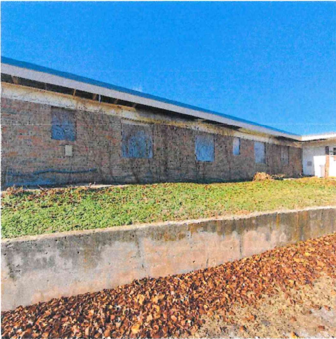
East Side Dec 2025 Mold on bricks
