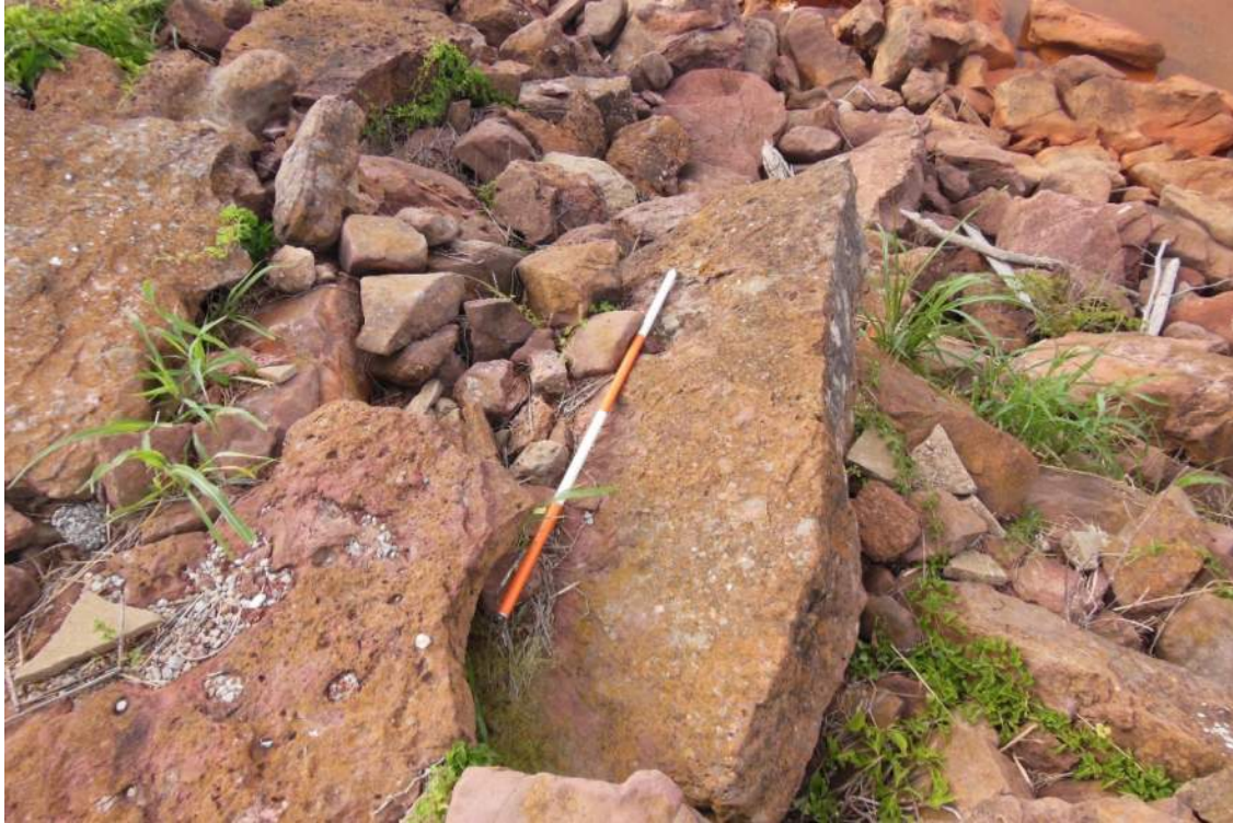
Photo No. 6: View of riprap on the upstream slope. Notice the mismatched sizes of rock and large sandstone slabs. The scale rod shown is 4ft long.
