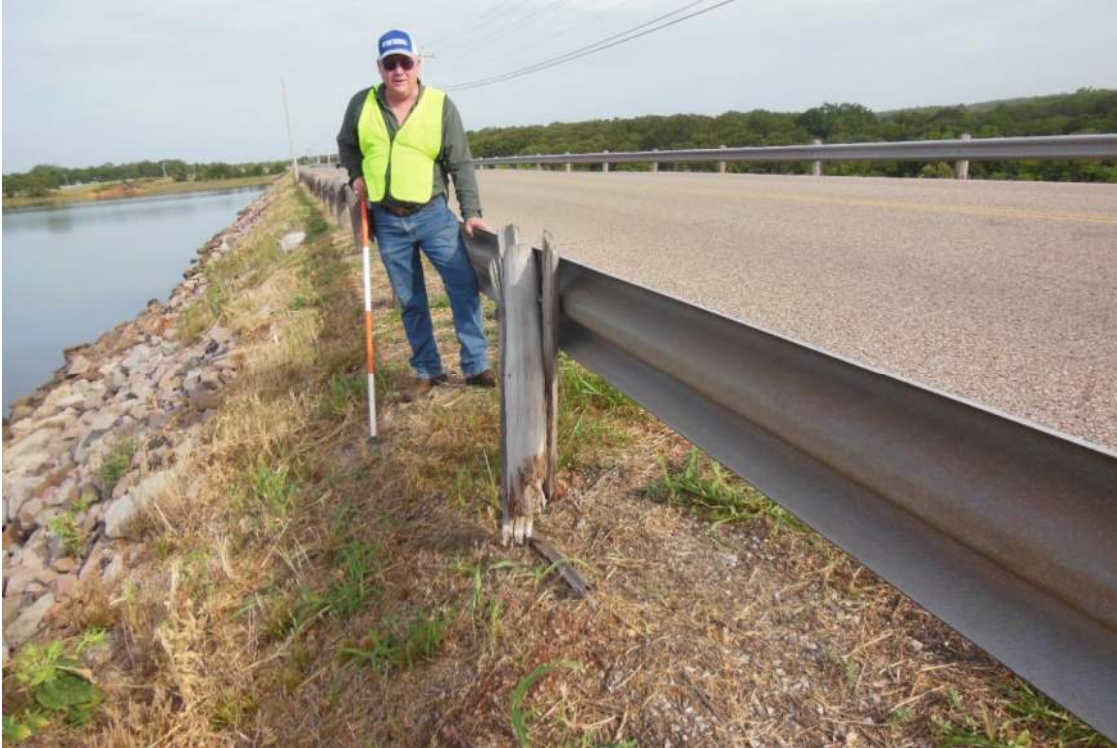
Photo No. 12: View of damage to guard rail post on the upstream side of the road.
