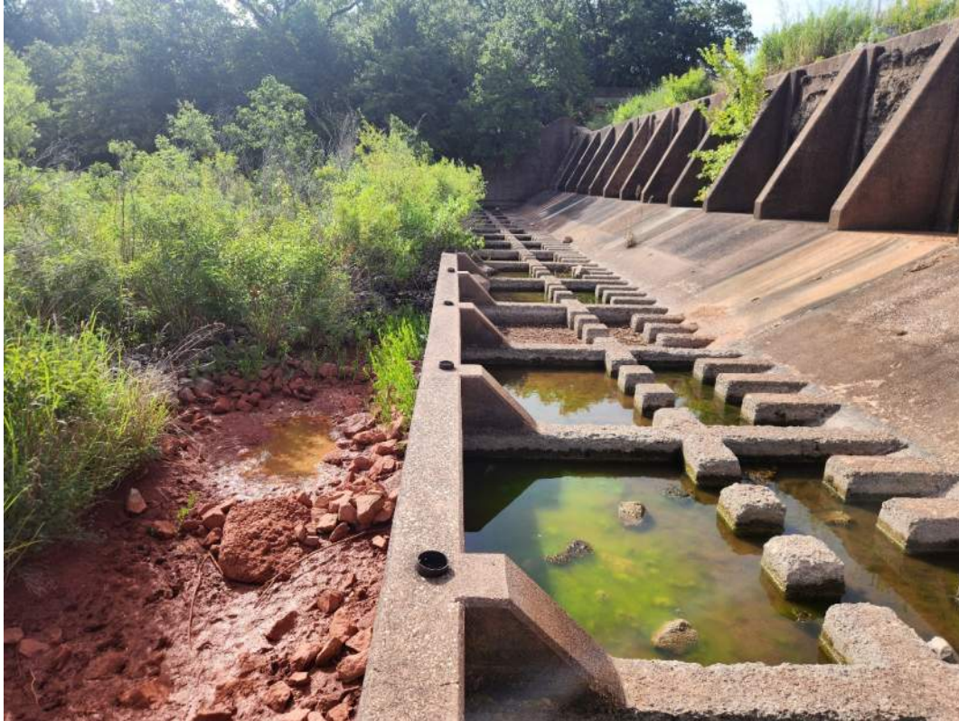
Photo No. 32: Downstream side of stilling basin structure. Some displaced riprap from previous flows noted downstream of end sill. Concrete surface weathering on energy dissipators.
