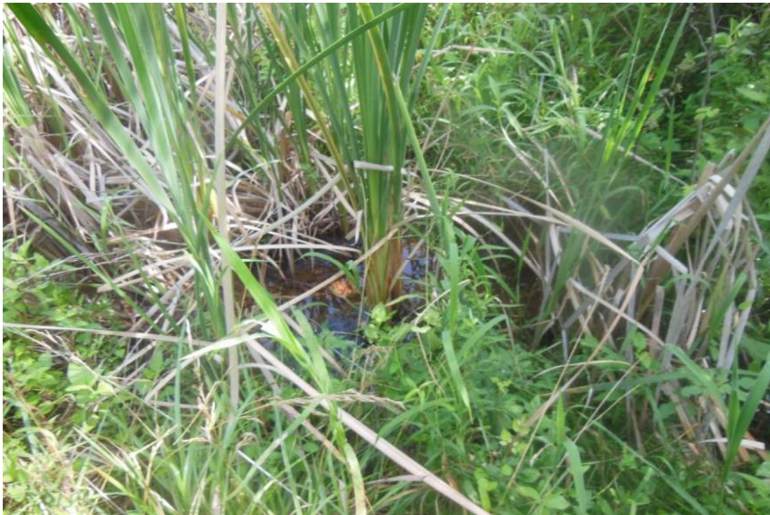
Photo No. 19: Typical view of standing water from seepage on the downstream toe near the abutments. The water was mostly clear and not visibly flowing.
