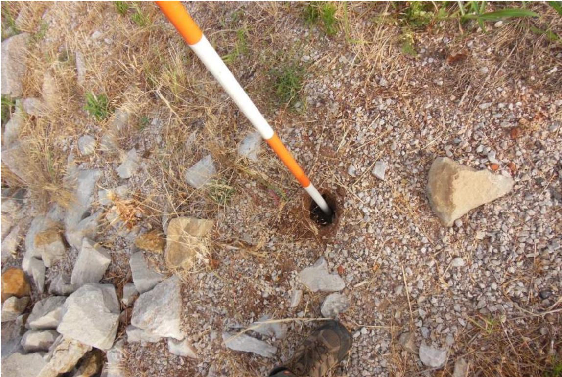
Photo No. 8: View of rodent hole on the upstream slope.
