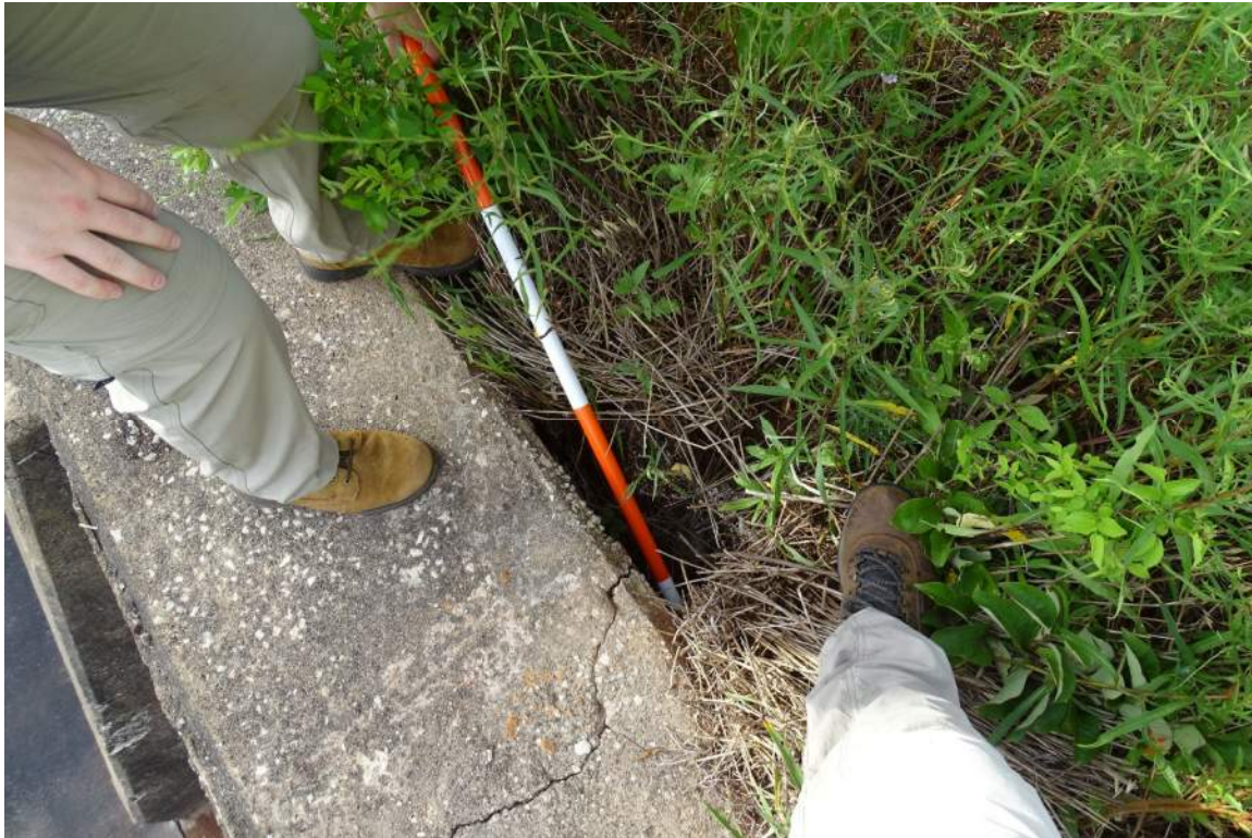
Photo No. 26: Additional scour upstream of the flip bucket walls.
