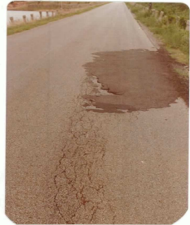
10. Pavement deterioration and subsequent repair.
