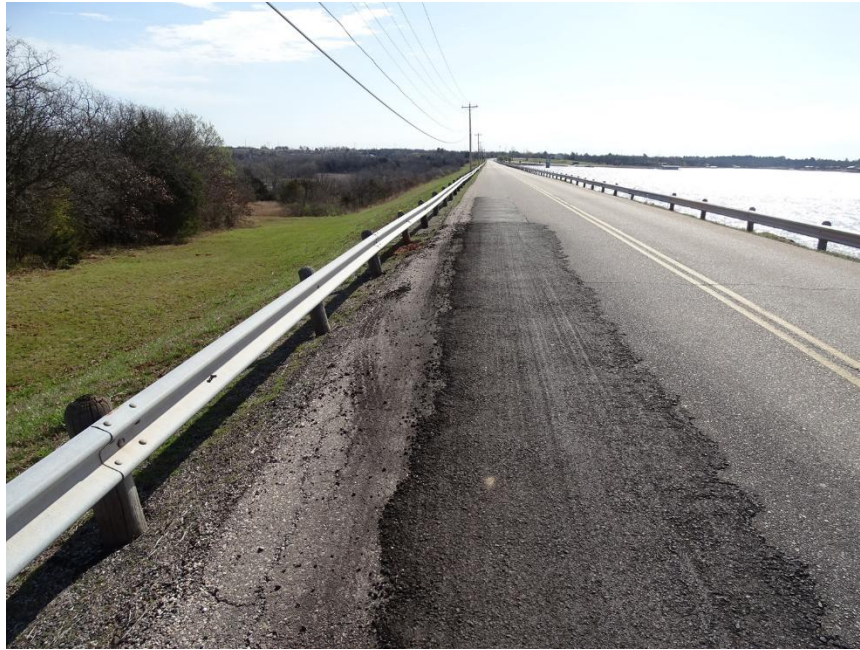
Figure 11. Road Repairs noted during the July 2024 inspection by FNI
