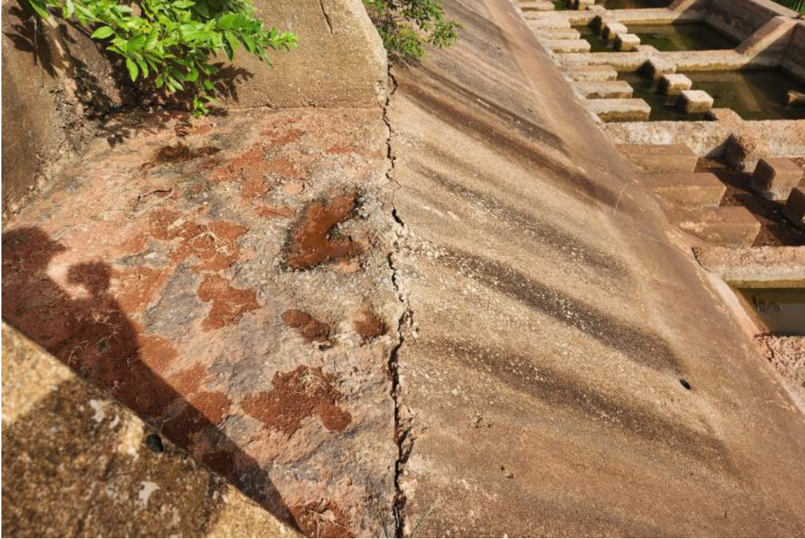
Photo No. 30: View of a concrete joint and some woody debris in the stilling basin.
