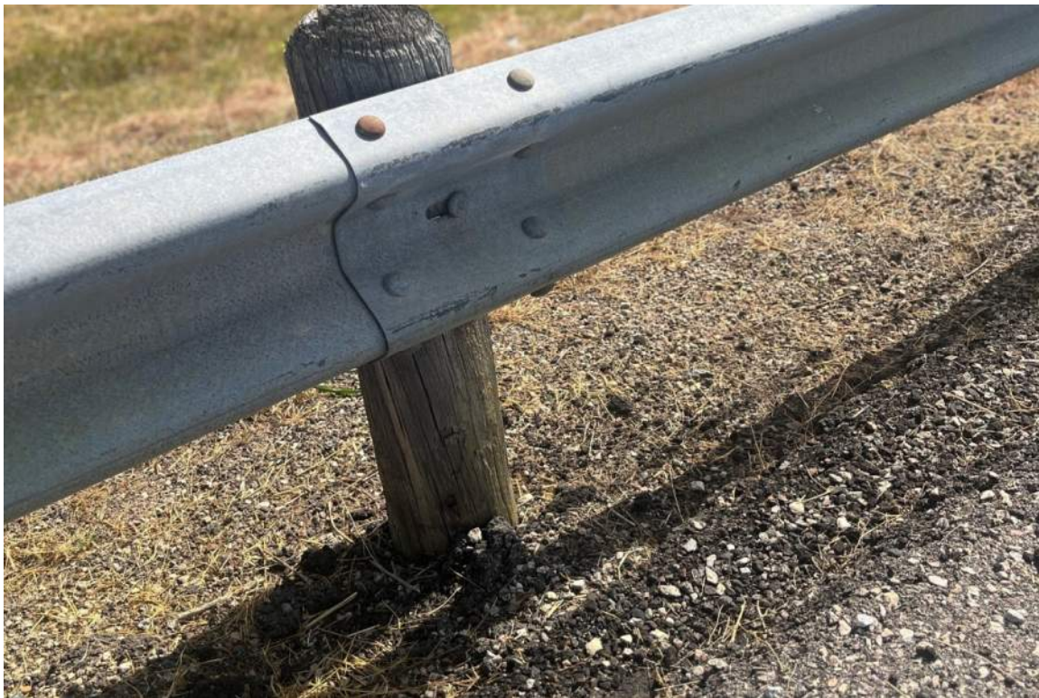
Photo No. 2: View of minor damage to guard rail along the crest of dam.
