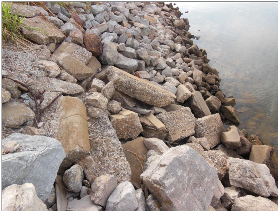
Figure 12. Armoring Repair – Mis-Matched Riprap
