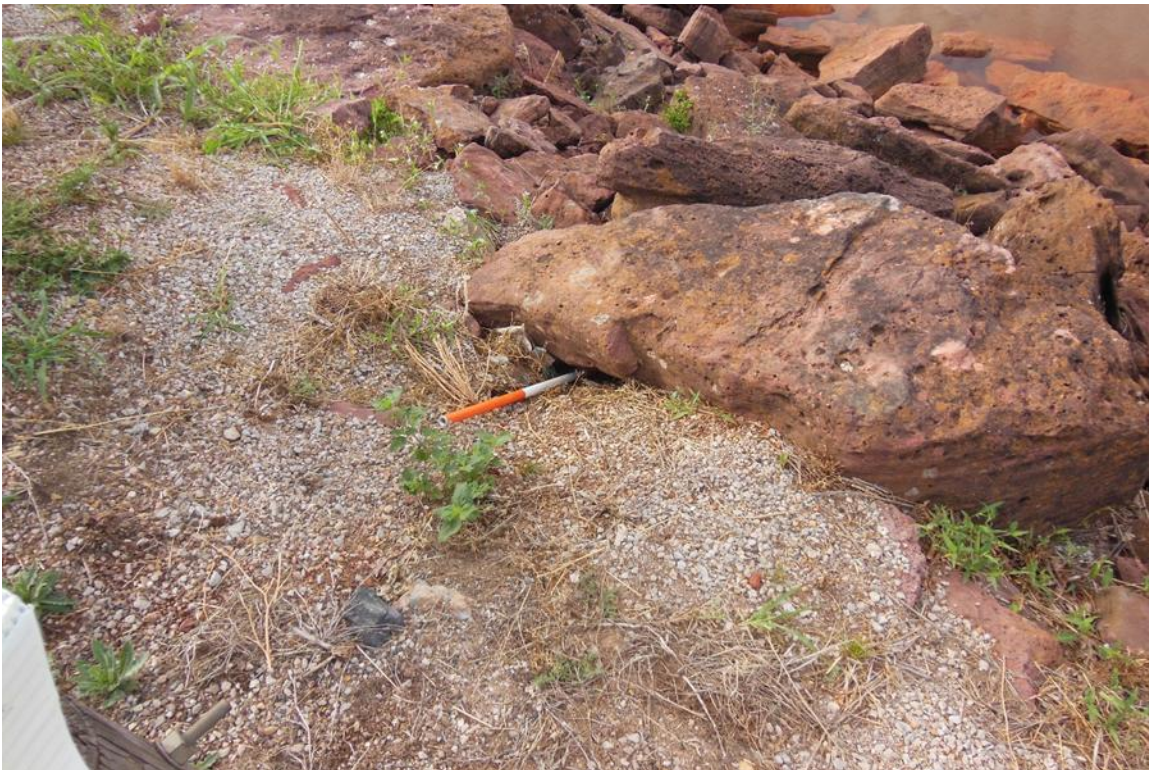
Figure 3. Mis-matched riprap and voids
