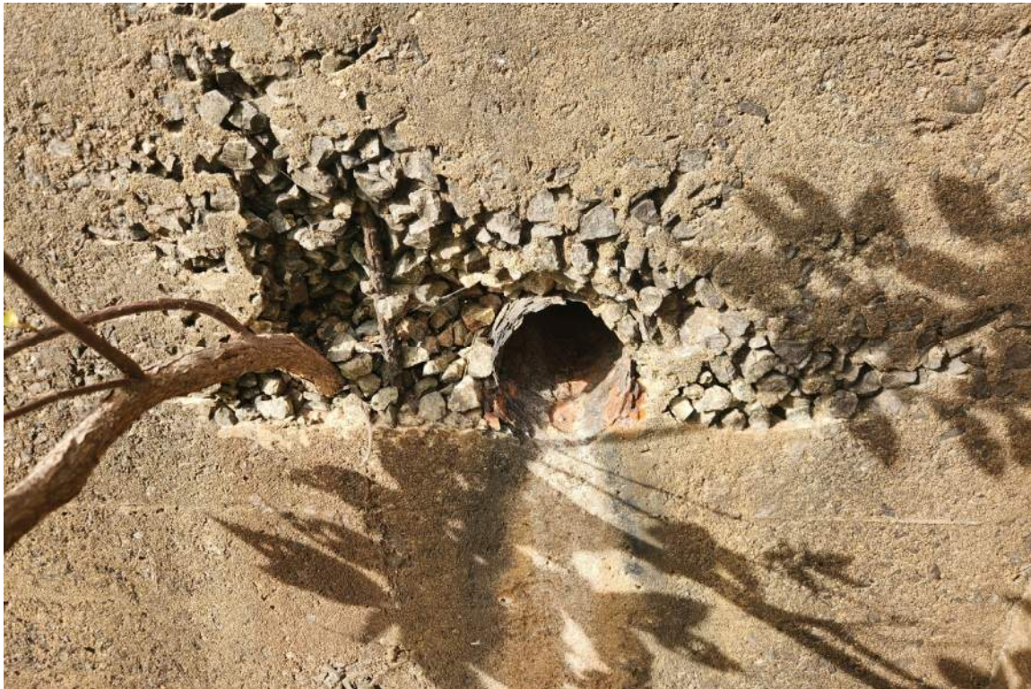
Photo No. 29: View of honeycombed concrete at base of back wall of flip bucket.
