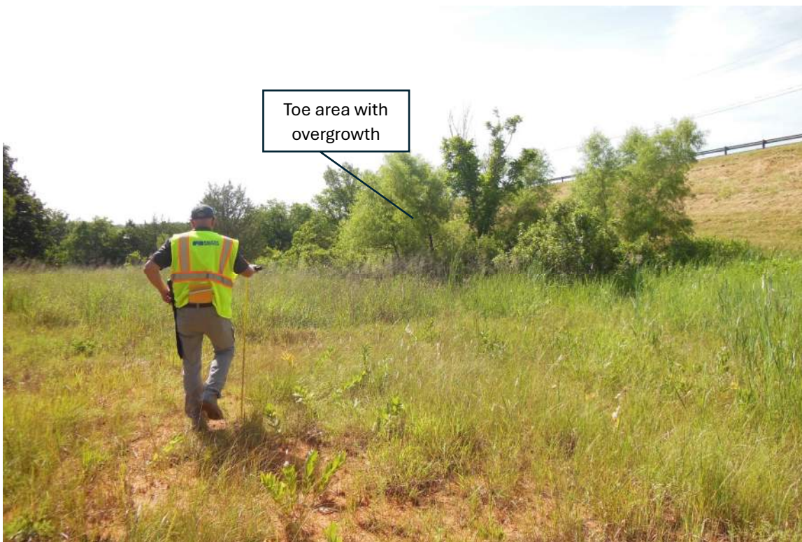
Photo No. 17: View of the downstream toe just east of the spillway. Notice the overgrowth along the toe.
