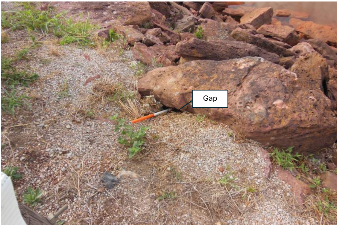
Photo No. 7: View of a gap under a large sandstone boulder near the crest of the slope. The gap has been created from washout of finer material under the large riprap.
