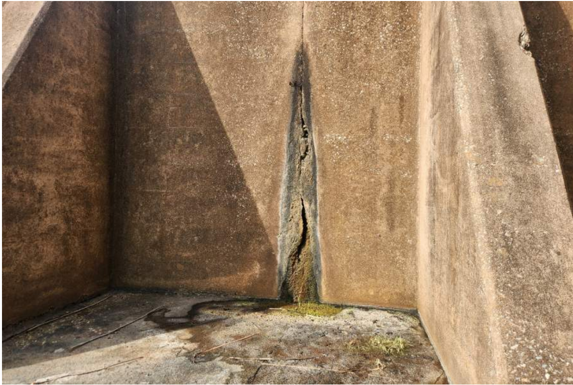
Photo No. 28: Some cracking and spalling along a concrete joint in one of the flip buckets.
