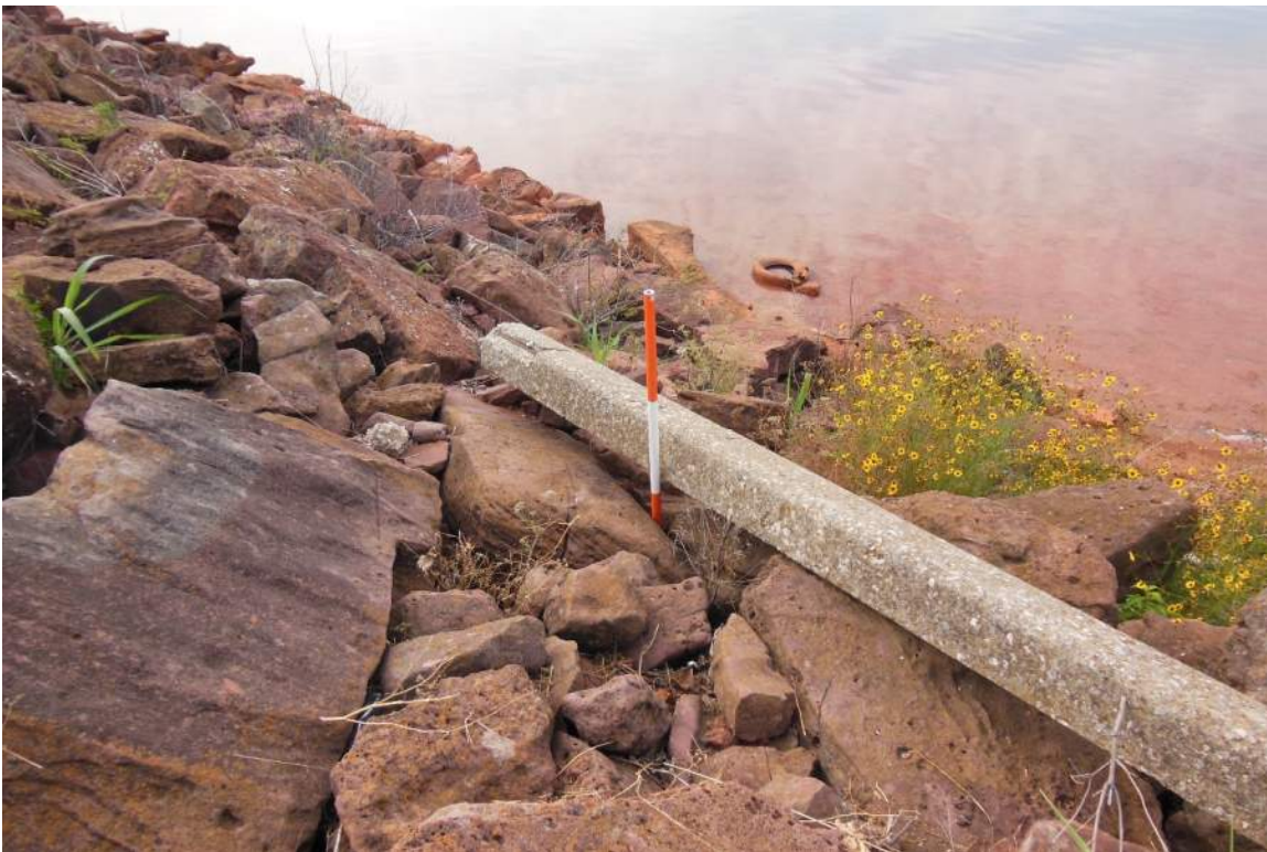
Photo No. 5: Photo of a large piece of concrete debris on the upstream slope. Rod is shown for scale.
