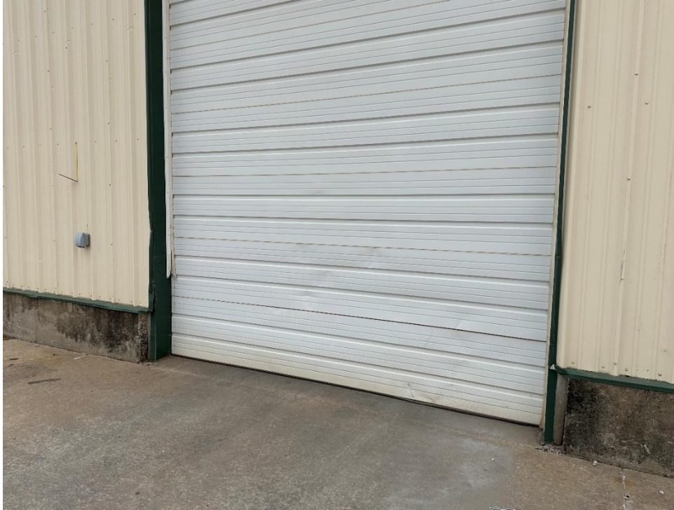
PHOTO #17: Damage to Over Head Door panels and building metal wall panels from flying debris.
