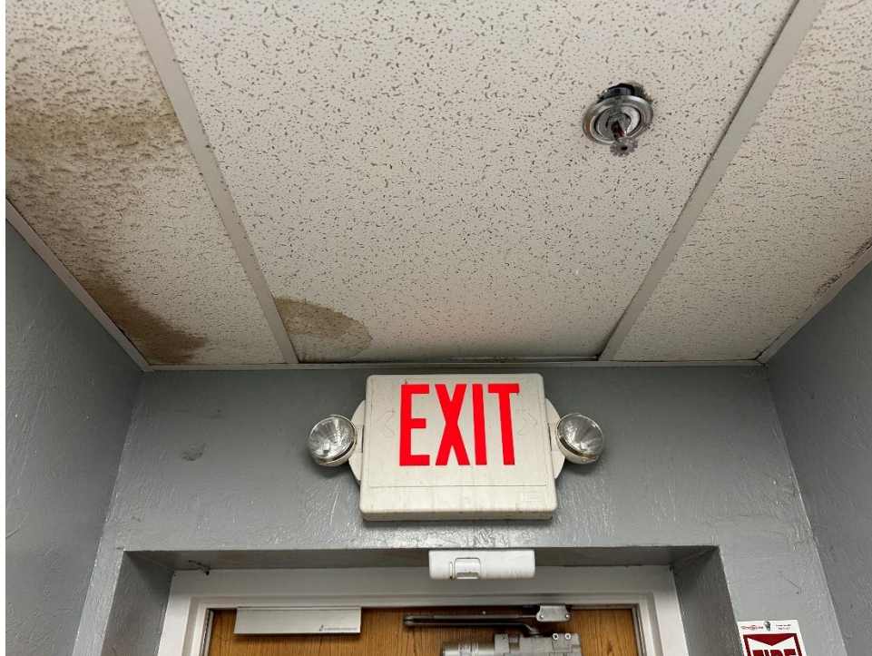
PHOTO #27: Close up of ceiling tile damage from water in hallway.
