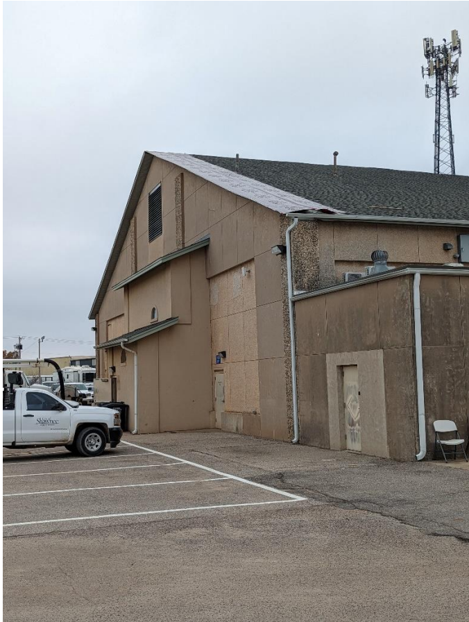
PHOTO #4: View looking northwest along south gable wall with roof damage.
