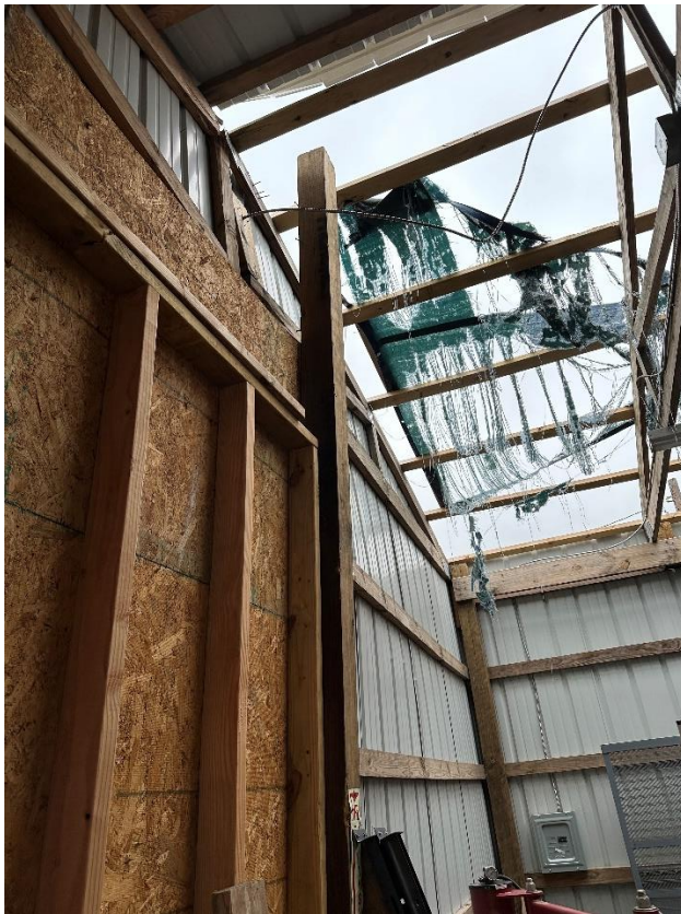
PHOTO #8: West end wood truss member and 6x6 wind column damaged.
