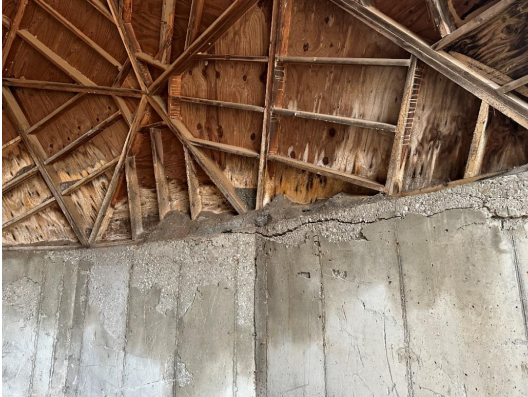
PHOTO #21: Damage to roofing, wood roof structure & concrete stem wall.
