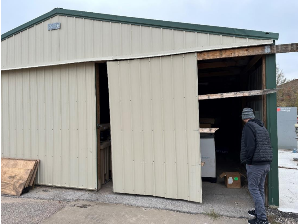
PHOTO #11: View of wood framed sliding door, metal panels, trim damaged.
