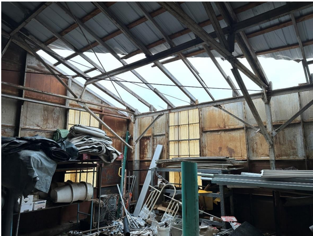
PHOTO #22: Damage to roofing, roof structural members at west wall.
