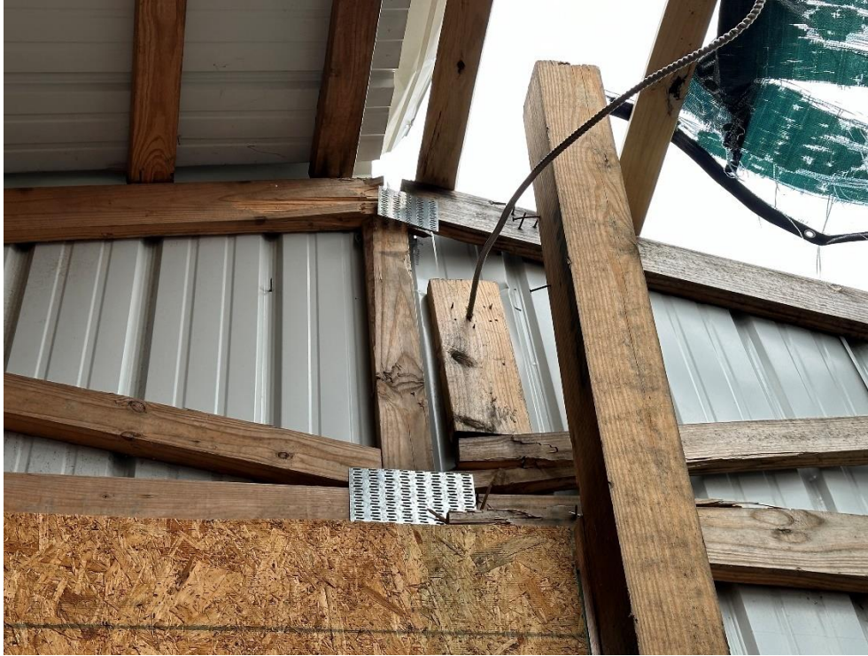
PHOTO #9: West end wood truss member and 6x6 wind column damaged.
