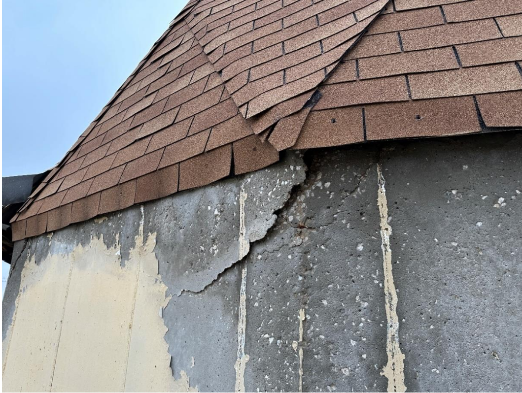
PHOTO #19: Damage to roofing, wood roof structure & concrete stem wall.
