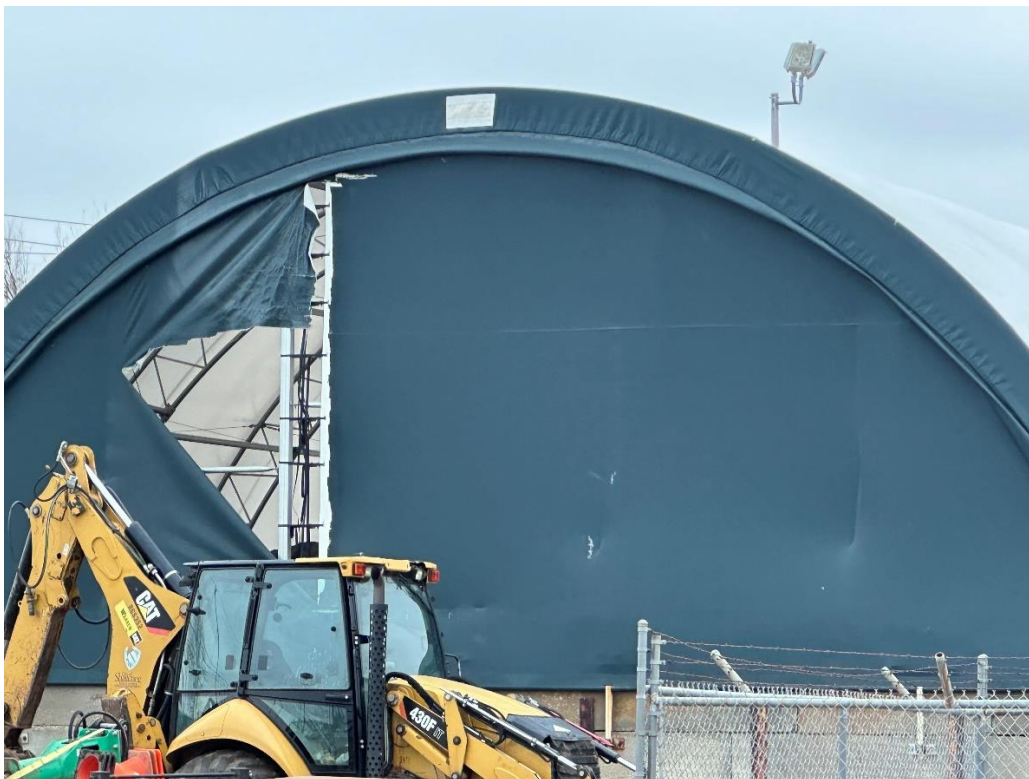
PHOTO #12: View of membrane structure fabric end wall damage.
