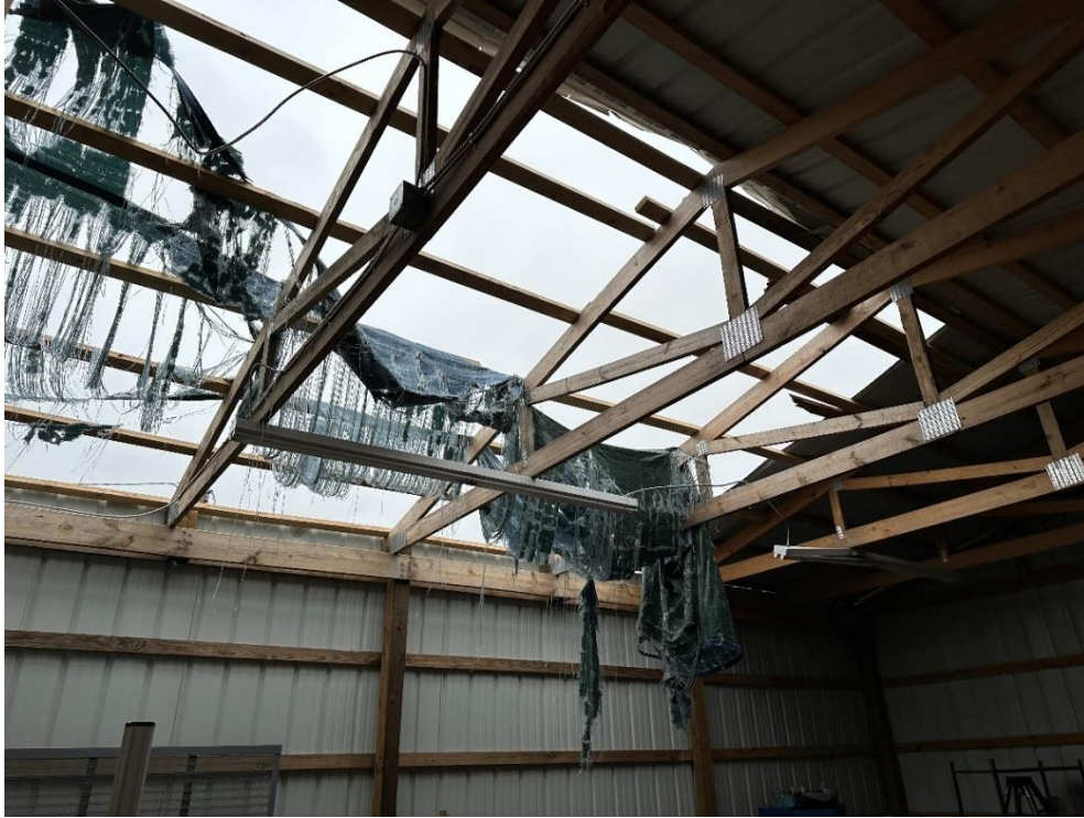
PHOTO #7: North side of roof partially removed with damaged 2x wood purlins.
