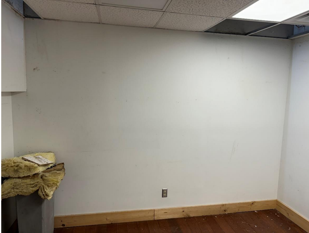
PHOTO #23: Water damage to south, east and west wall due to exposure to elements for months.
