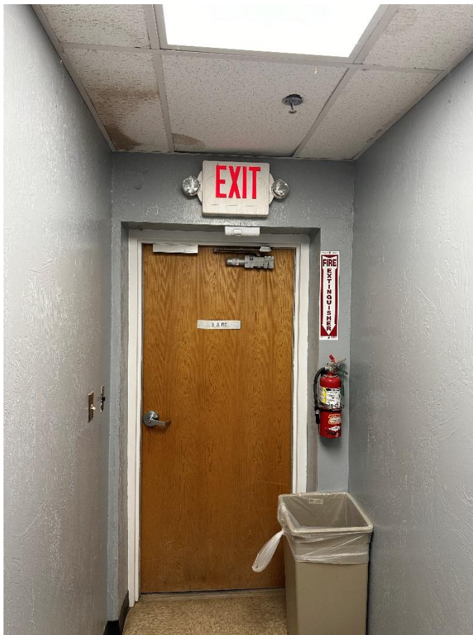
PHOTO #26: Damage to ceiling tile in hallway above door to exit stair.
