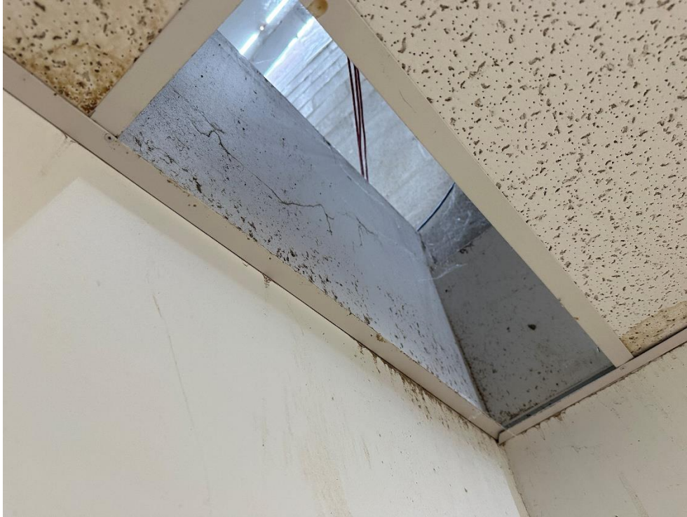
PHOTO #29: Close up of open area exposed to water damage area.
