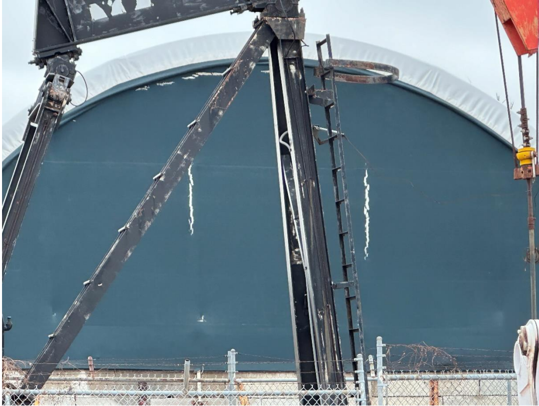
PHOTO #13: View of membrane structure fabric end wall damage.
