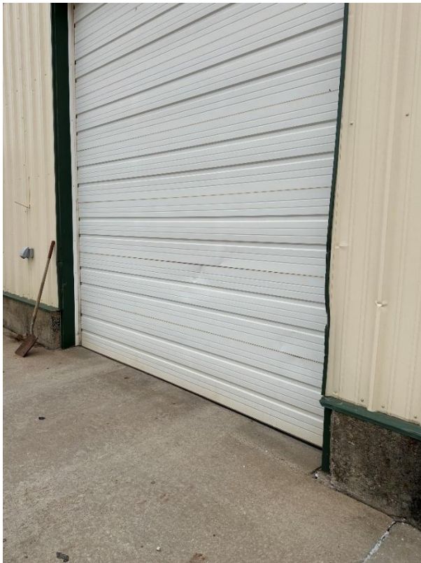
PHOTO #16: Damage to Over Head Door panels and building metal wall panels from flying debris.
