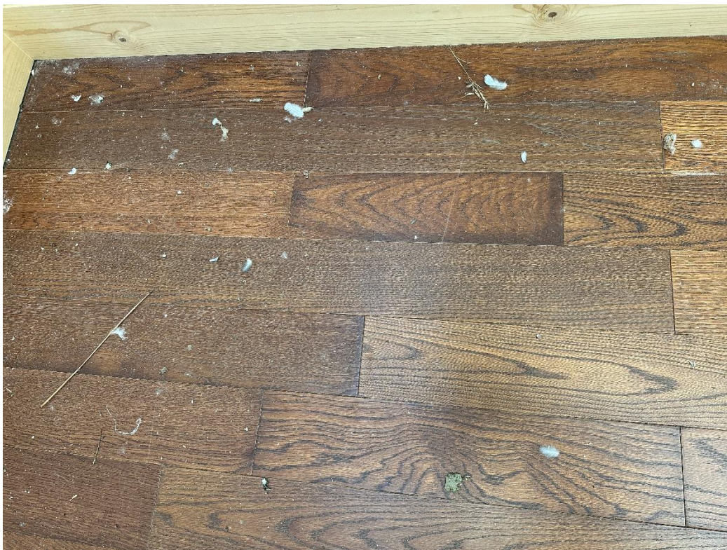
PHOTO #24: Flooring has buckled due to excessive exposure to water.
