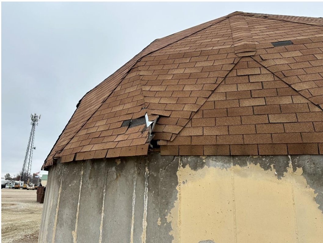
PHOTO #18: Damage to roofing, wood roof structure & concrete stem wall.
