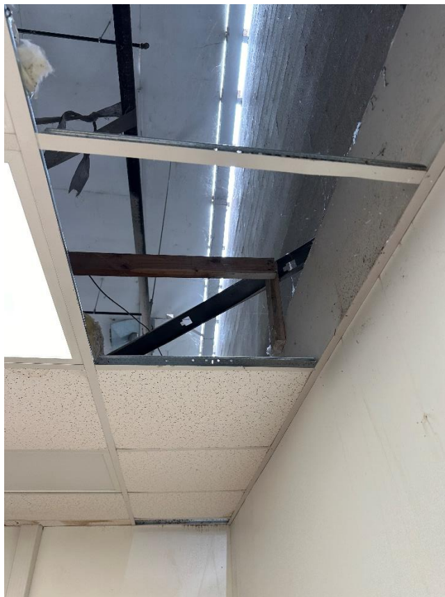
PHOTO #28: Open roof for a period of time over the office area that caused the water damage.
