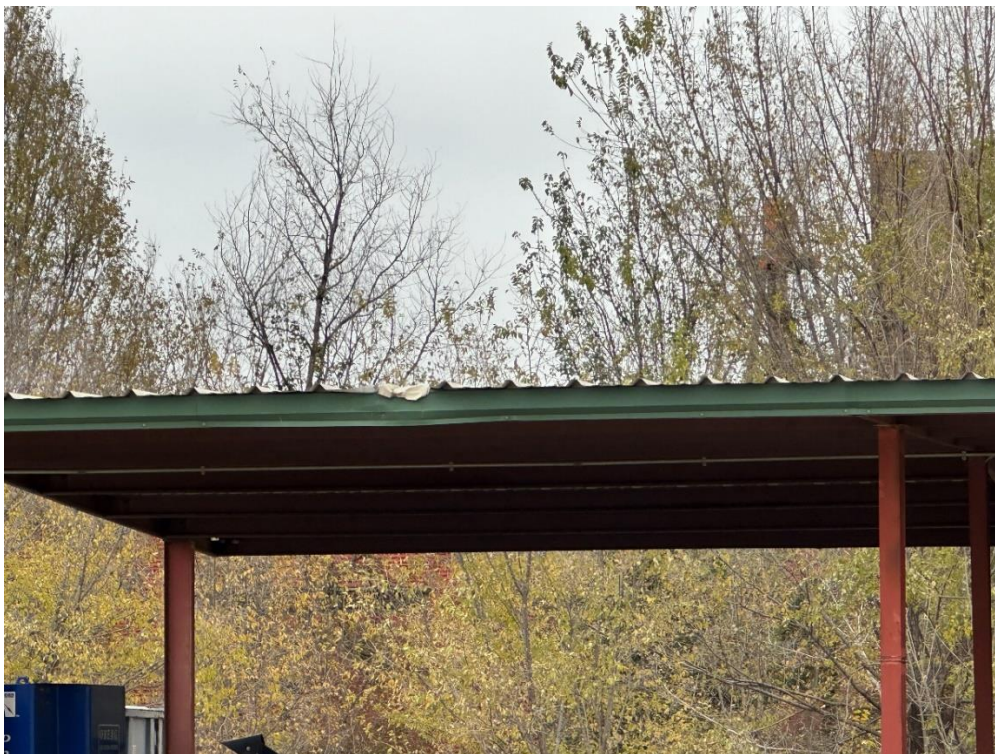
PHOTO #14: Damage to roof and metal trim from flying debris at canopy structures.
