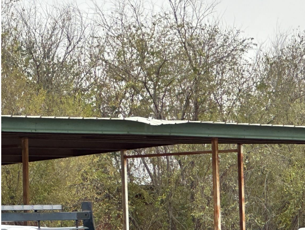
PHOTO #15: Damage to roof and metal trim from flying debris at canopy structures.
