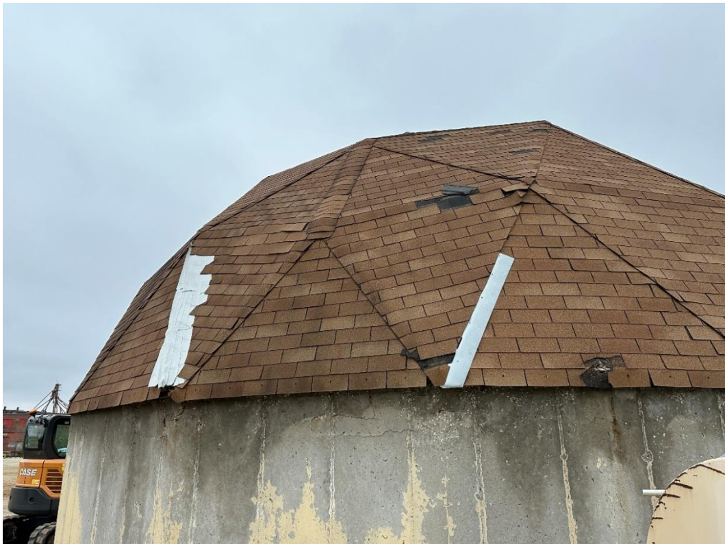
PHOTO #20: Damage to roofing, wood roof structure & concrete stem wall.
