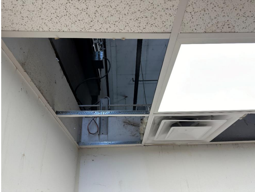
PHOTO #25: Damage to ceiling tile from water exposure for months.
