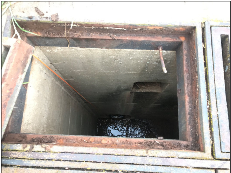
Figure 3: Inside of Grate Inlet Showing Void Requiring Filling
