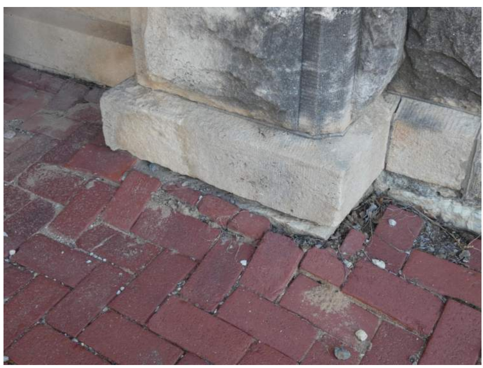
A EXISTING CONDITIONS PHOTO NOT TO SCALE
