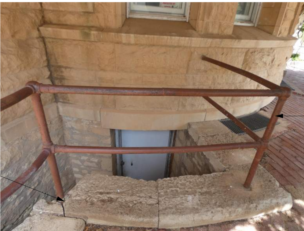
A EXISTING CONDITIONS PHOTO NOT TO SCALE
