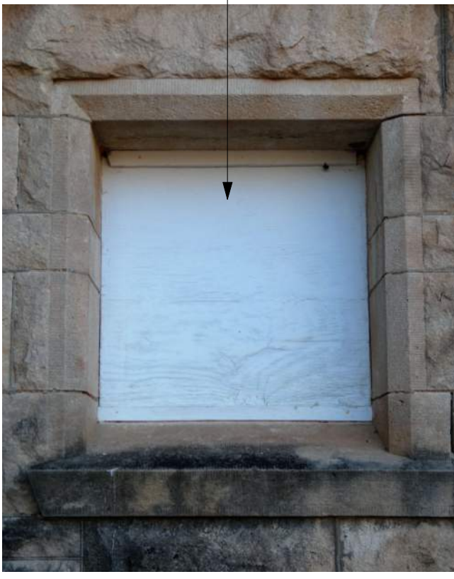
BOARDED UP WINDOW (EAST SIDE)
