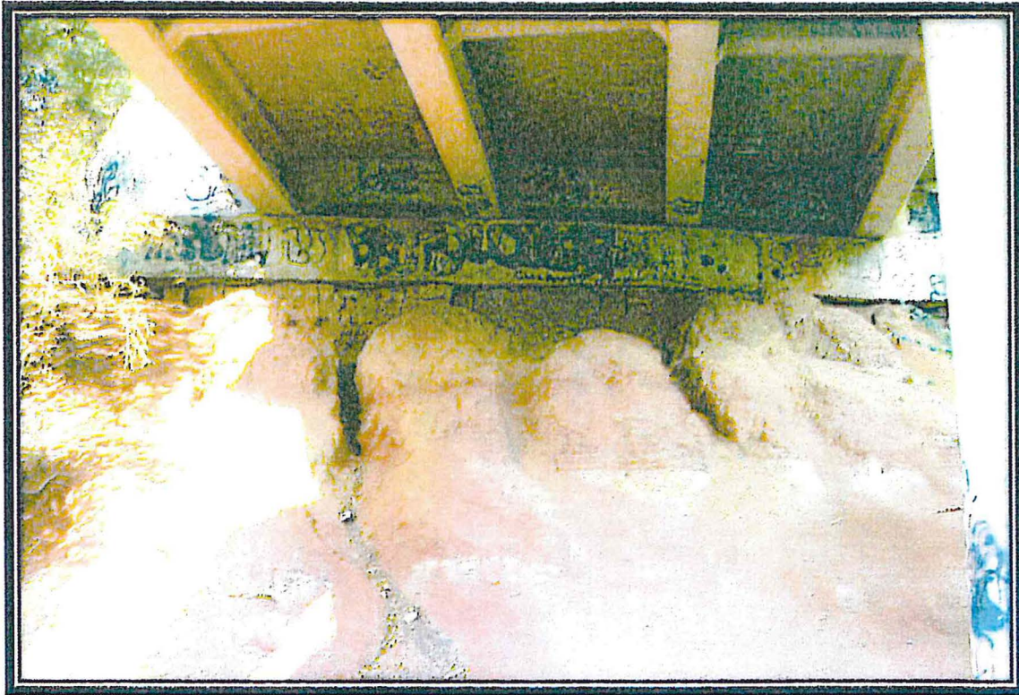
Erosion at East Abutment, West is similar
