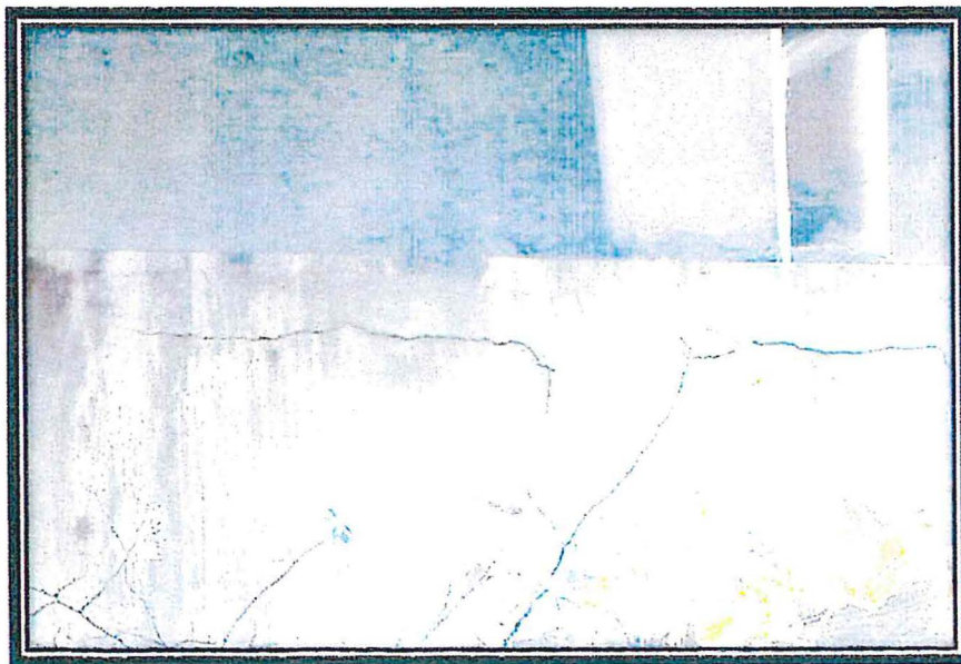
Cracks on West Pier Cap
