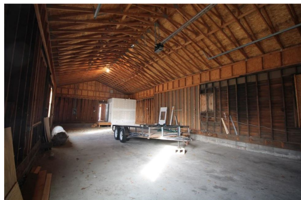
Picture D- Equipment room - interior
