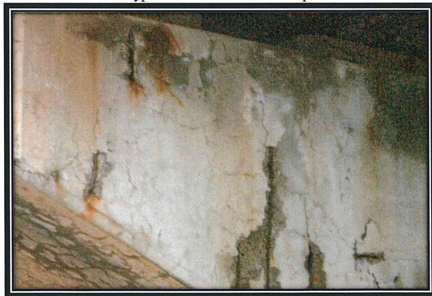
Another Pier Cap showing Typical Conditions
