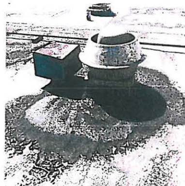
Surface debris around penetration
