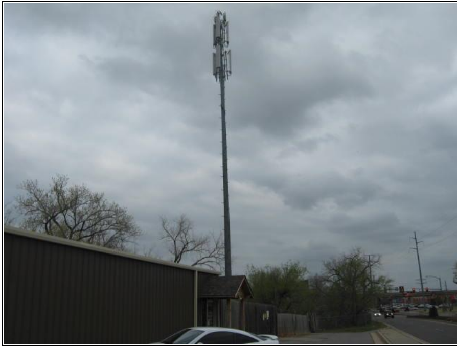
Photo of monopole at 5420 N Belle Isle Blvd
