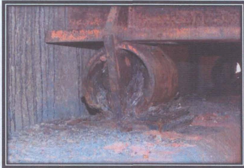
Condition of Worst Roller Bearing
