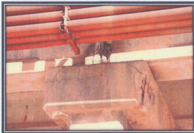
Spalling at Beam Ends
