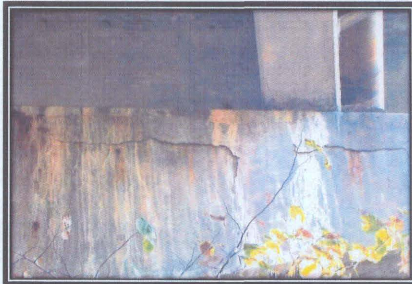
Cracks on West Pier Cap
