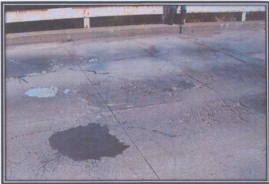
Deteriorated Area of 2" Concrete Overlay
