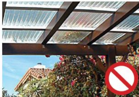
Corrugated plastic is not acceptable
