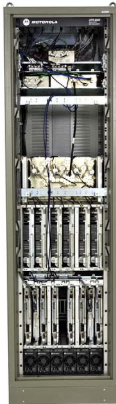
Figure 1-5: General GTR ESS Front View
